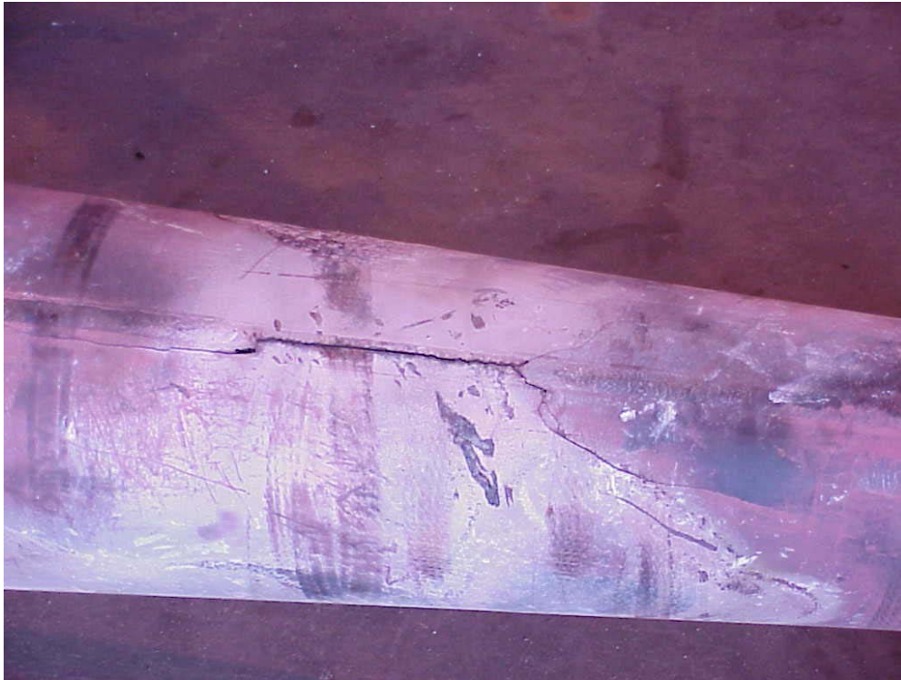
Figure 12.13: Crack Along Longitudinal Seam of Thermo Compressor Cone
